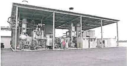
1 × 1,320 kW at rubber factory
