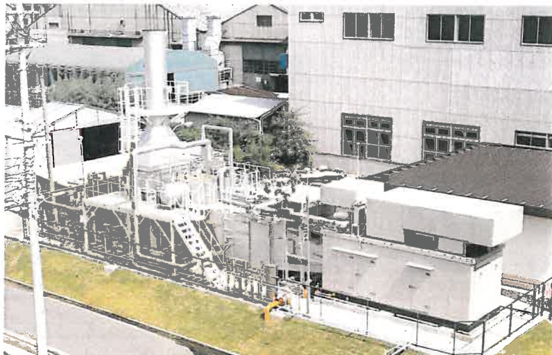
1 × 2,000 kW Cheng-cycle system at turbine factory
