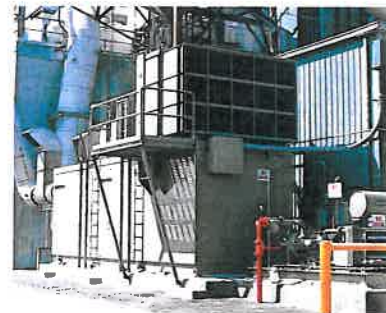
1 × 1,400 kW at soap-powder factory
