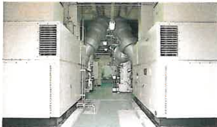
2 × 500 kW at chemical factory
