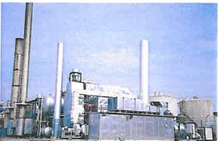
1 × 1,350 kW at chemical factory
