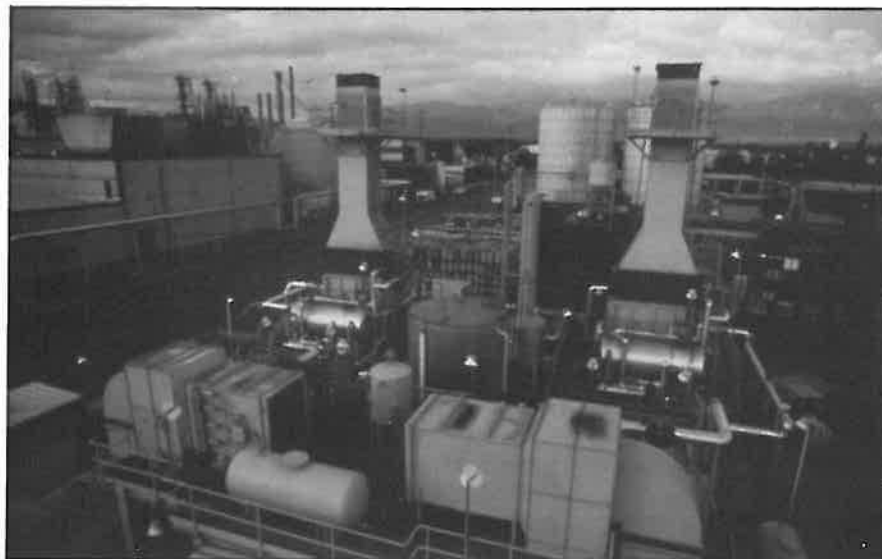
This Cheng Cycle Series 7 cogeneration plant at Sunkist Growers in Ontario, California, U.S.A., was the second of six current Cheng Cycle installations in California.
