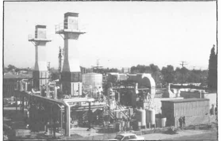
Figure 7. Sunkist growers' installation
