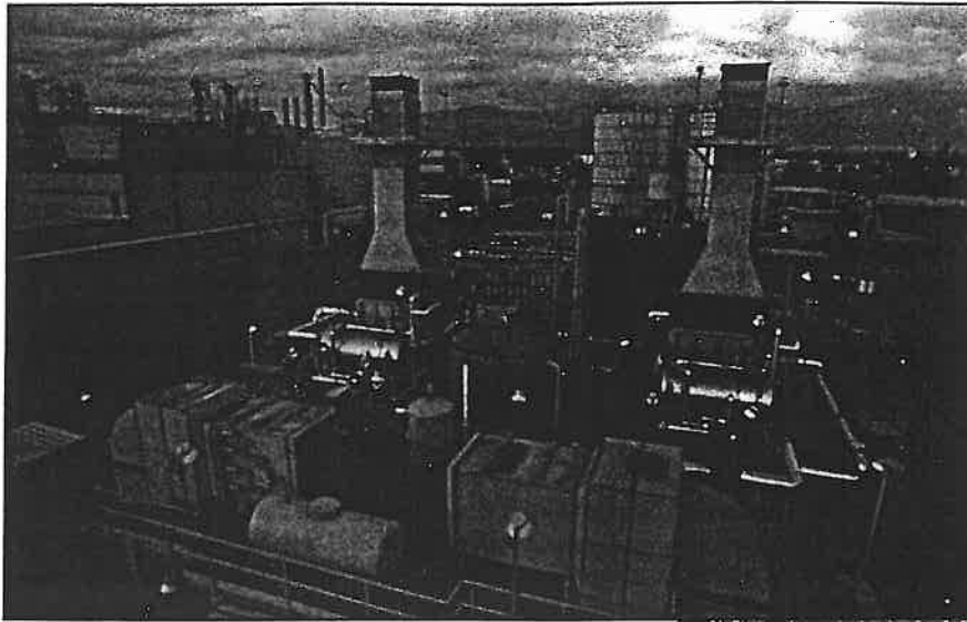
This Cheng Cycle Series 7 cogeneration plant at Sunkist Growers in Ontario, California, U.S.A., was the second of six current Cheng Cycle installations in California.
